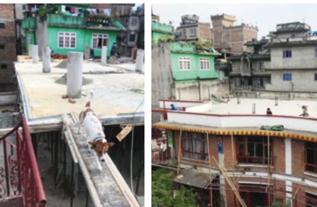
Construction site at the main center of Shanti Leprosy Relief in Kathmandu's Tilganga district. New classrooms are being built here.
